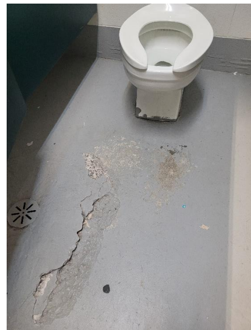
Photo 12 – Damaged Slab in Washroom
