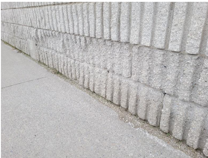
Photo 23 – Damaged Split Ribbed Block at Southeast Corner
