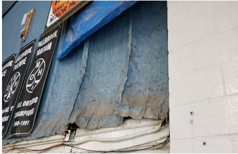
Photo 013 Significant Damage to Metal Cladding
