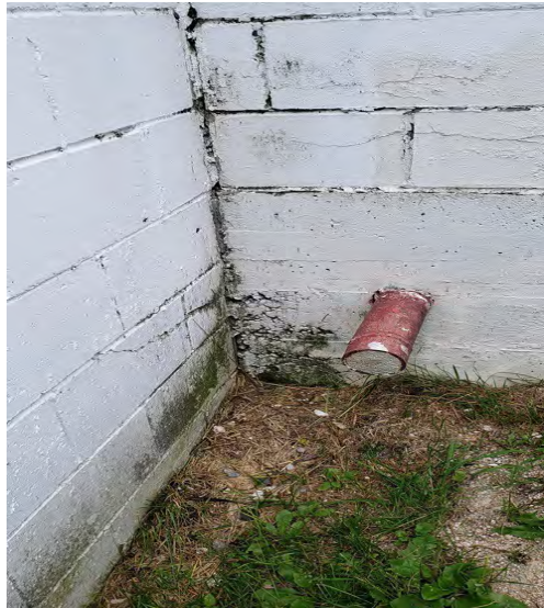
Photo 082 Honeycombing and Mould Growth
