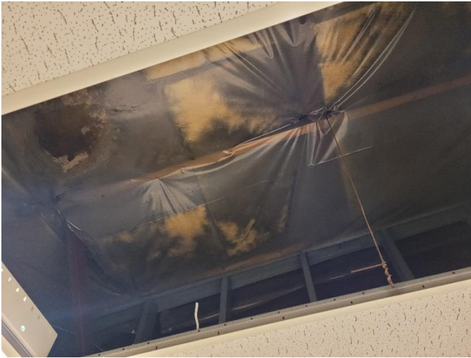
Photo 17 – Mould and Evidence of Moisture
