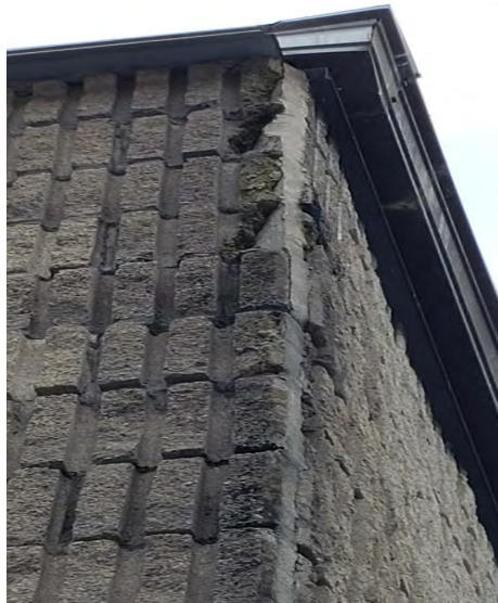
Photo 067 Localized Block Damage at South-East Corner
