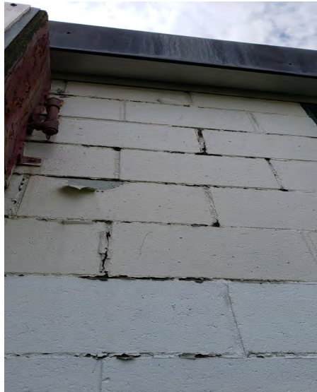
Photo 080 Step Cracking and Paint Peeling
