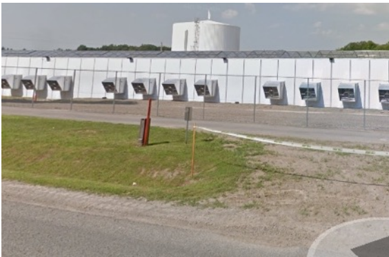
Ventilation equipment on east side of CannTrust Facility in the Town of Pelham (Source: Google)
