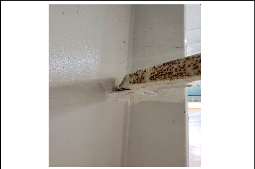
Photo 004 Rust on Frame Brace
