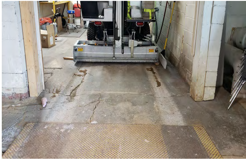
Photo 020 Resurfacing Room Rutting
