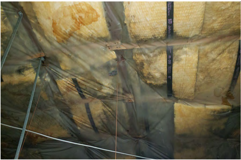
Photo 060 Moisture in Roofing System
