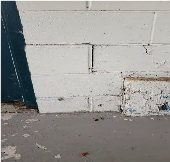
Photo 039 Step Cracking and Damage to West-Side Exit
