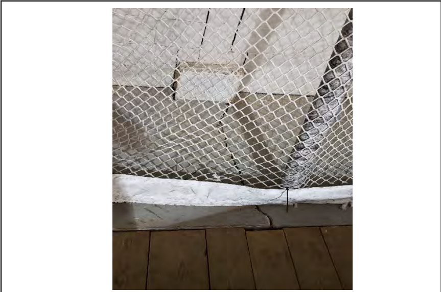
Photo 024 Cracking Under North-Side Column
