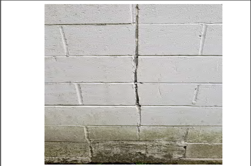
Photo 091 Damaged Wall Joint
