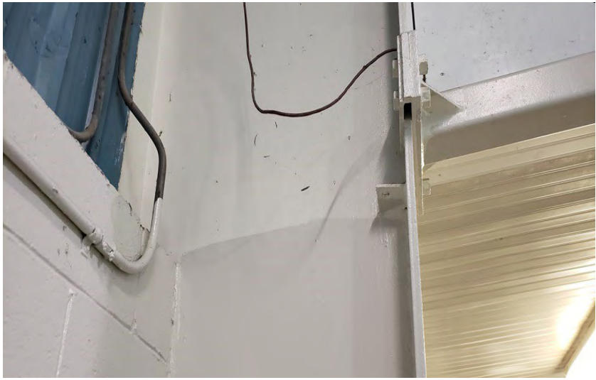
Photo 008 Missing Brace at Southmost Frame
