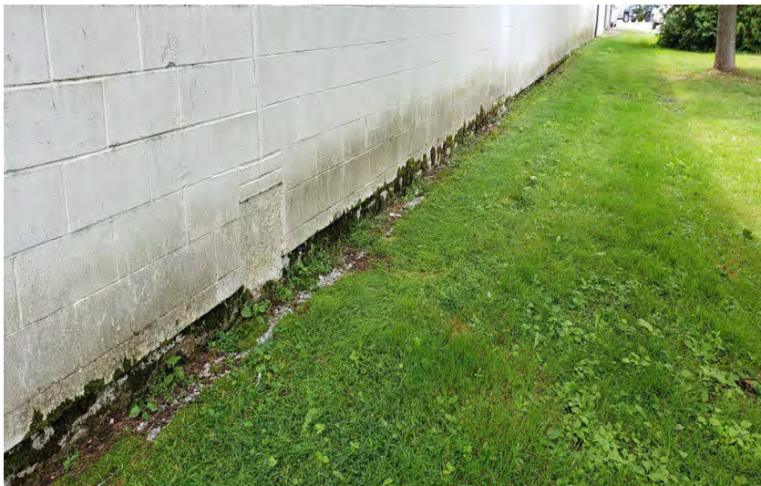
Photo 090 Mould Along West Side
