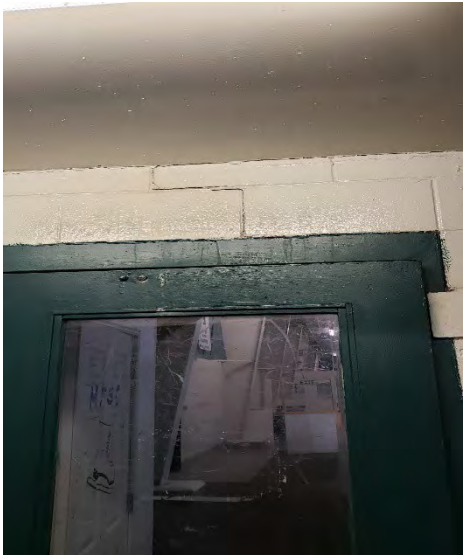
Photo 030 Step Cracking in Lobby
