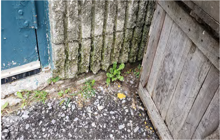
Photo 074 Deterioration of Blocks
