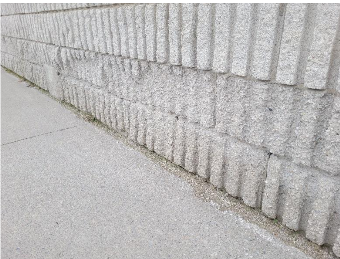
Photo 23 – Damaged Split Ribbed Block at Southeast Corner
