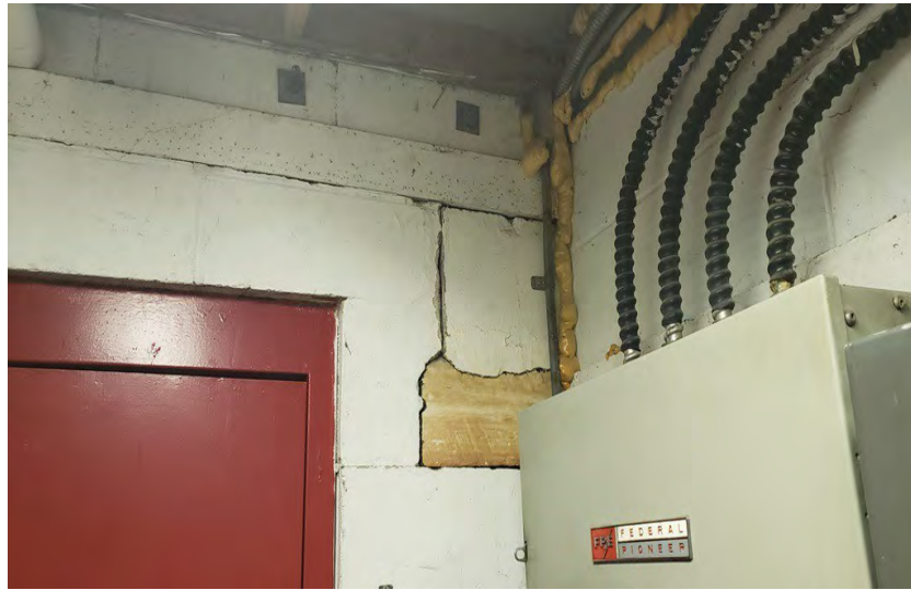
Photo 035 Wooden Block Replacement and Cracking
