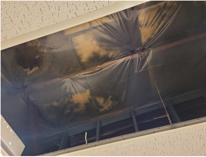
Photo 17 – Mould and Evidence of Moisture
