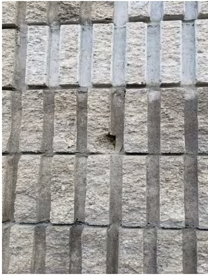
Photo 066 Localized Brick Damage
