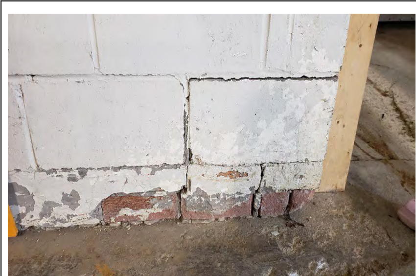
Photo 038 Block and Joint Damage
