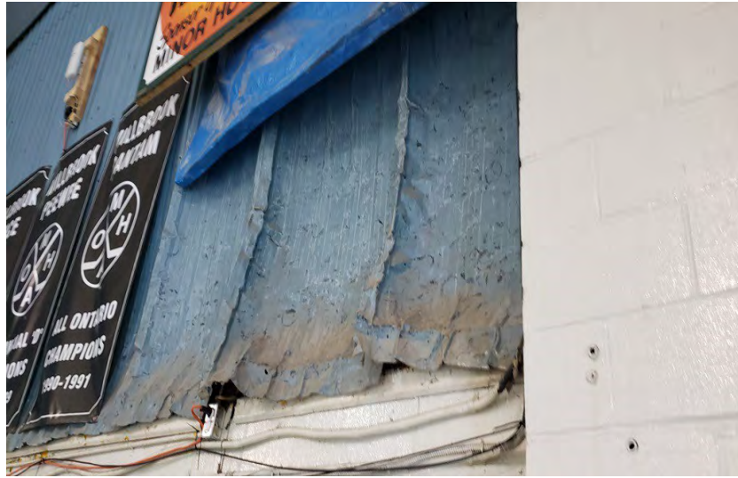
Photo 013 Significant Damage to Metal Cladding
