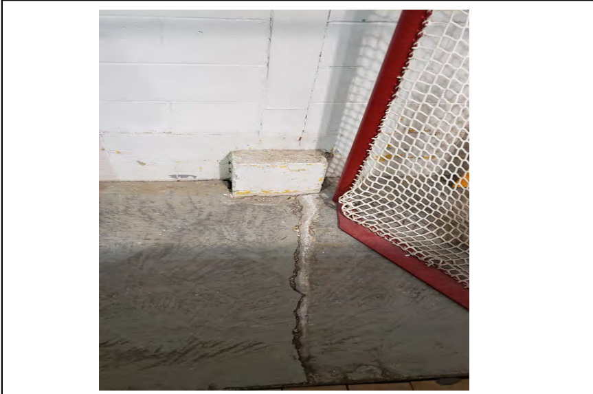
Photo 023 Cracking Under North-Side Column
