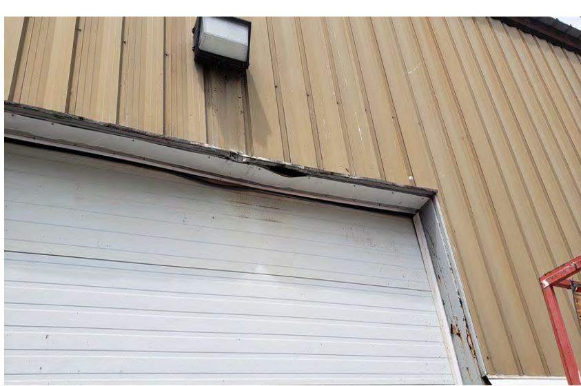
Photo 077 Damage to Garage Door Opening
