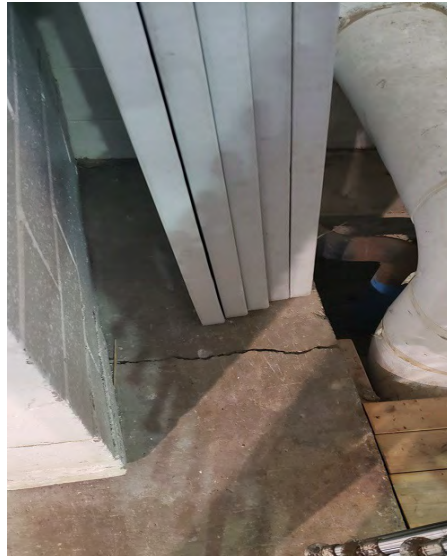
Photo 019 Major Crack in Apron Slab
