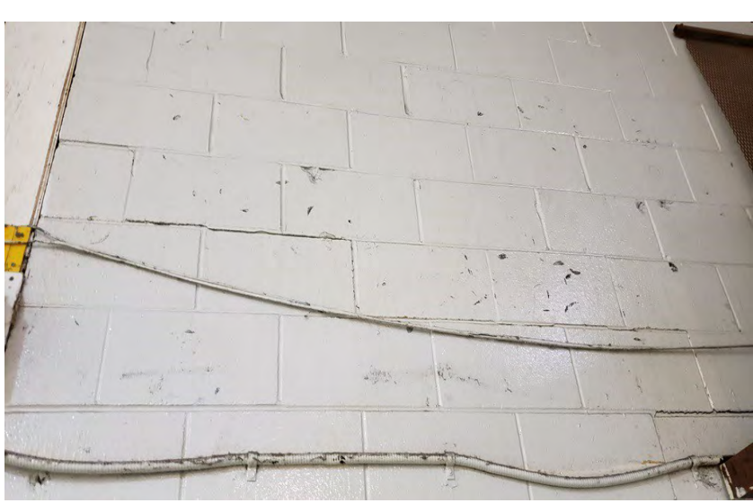
Photo 029 Step Cracking Along South-Face Wall
