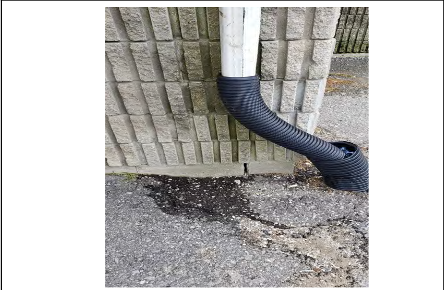
Photo 071 Gap in Foundation Wall
