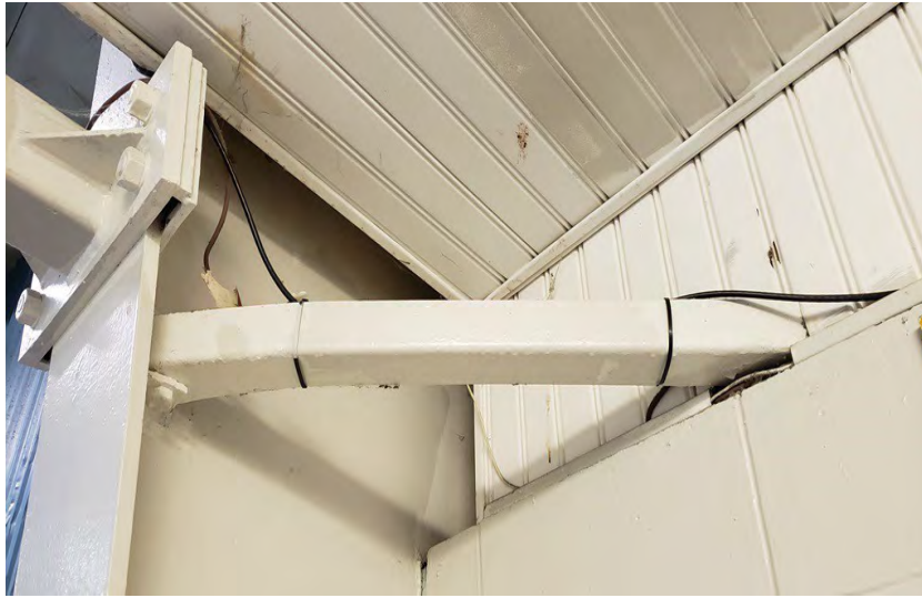
Photo 009 Bent Braced member
