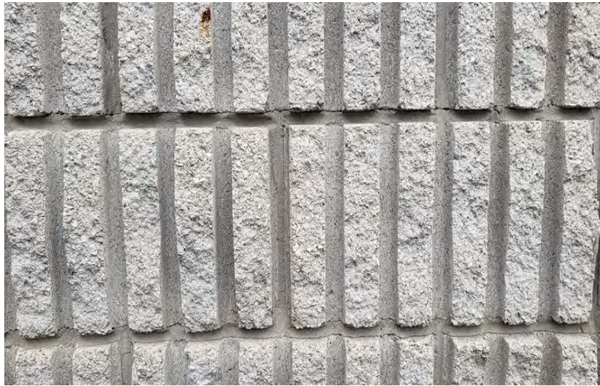
Photo 065 Architectural Block Mortar Cracks
