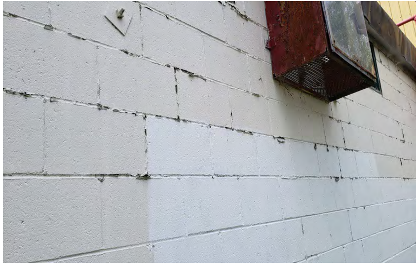
Photo 079 Step Cracking and Paint Peeling
