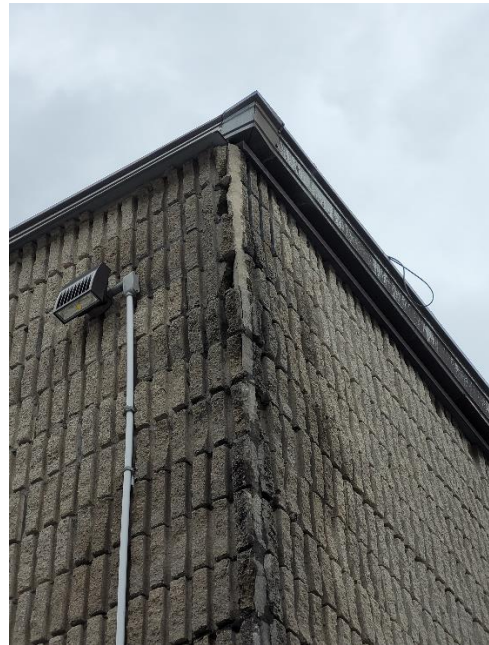
Photo 22 – Damaged Split Ribbed Block at Southeast Corner
