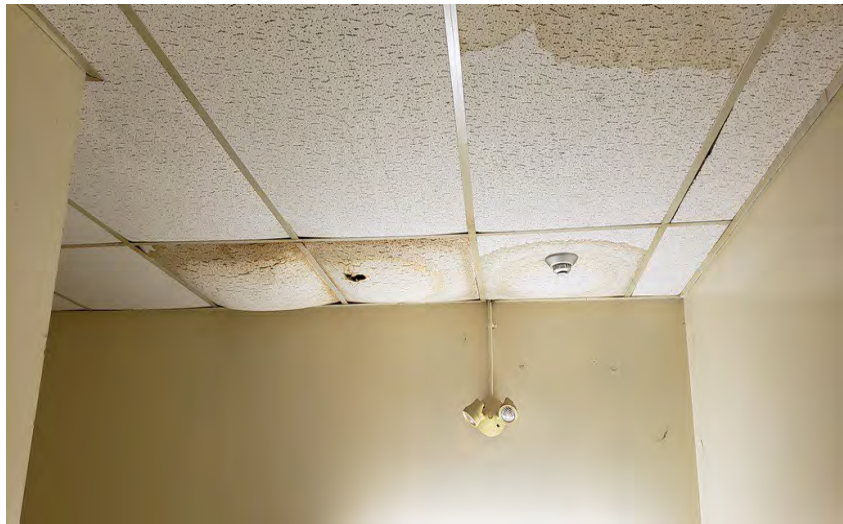
Photo 061 Signs of Moisture Damage
