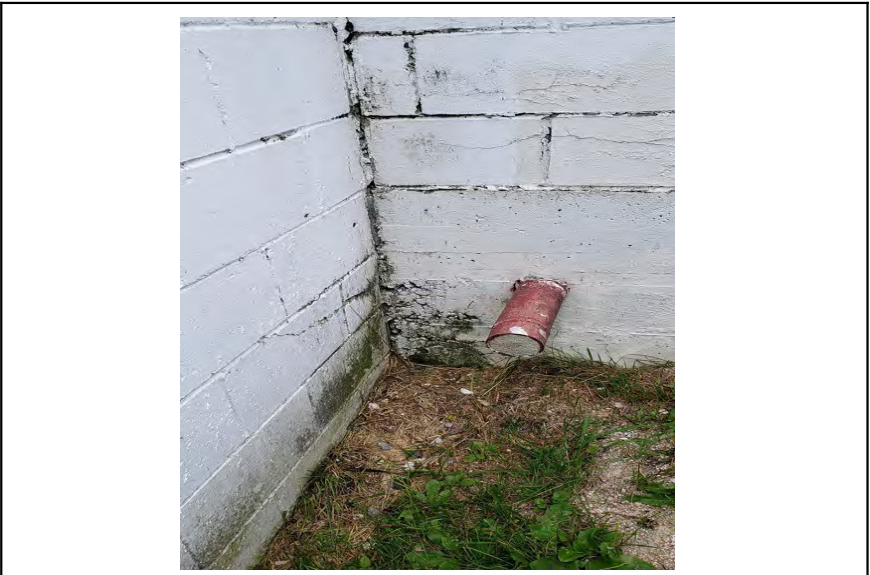
Photo 082 Honeycombing and Mould Growth
