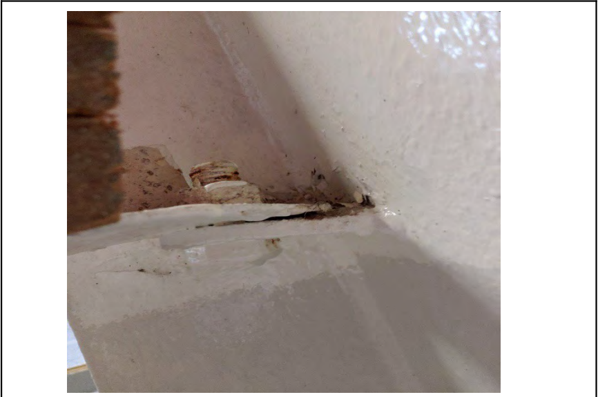
Photo 006 Rusted Bracing Connection
