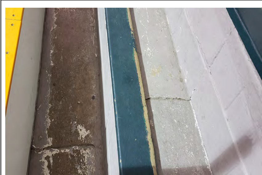
Photo 011 Bleacher Crack at Joint Location
