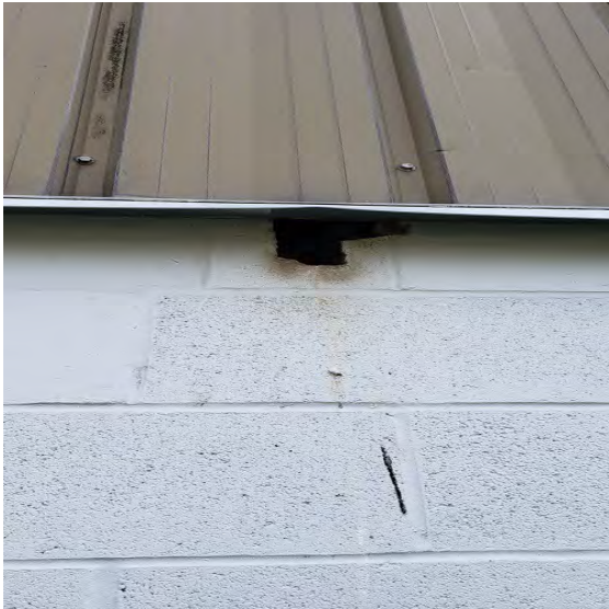
Photo 093 Hole in Masonry Block
