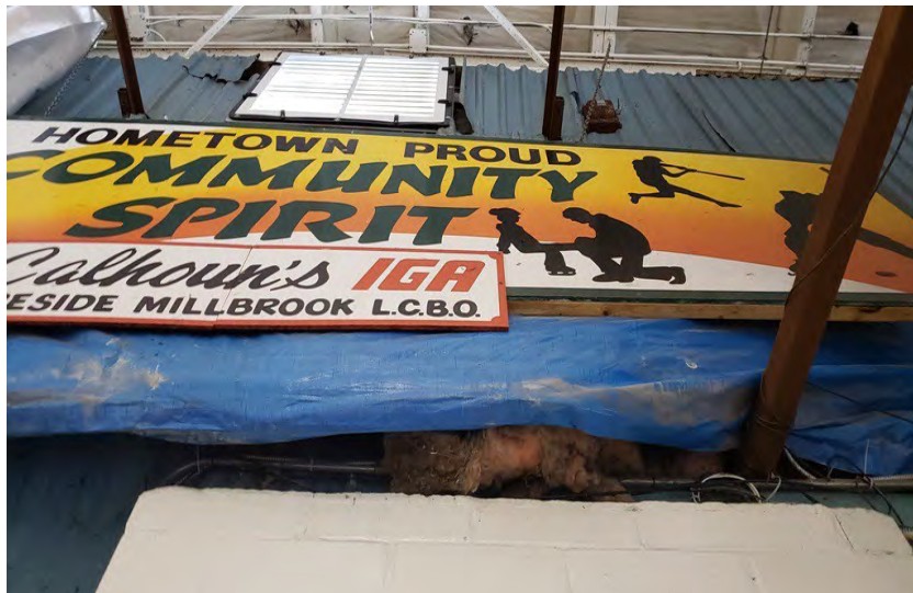
Photo 014 Metal Cladding Damage
