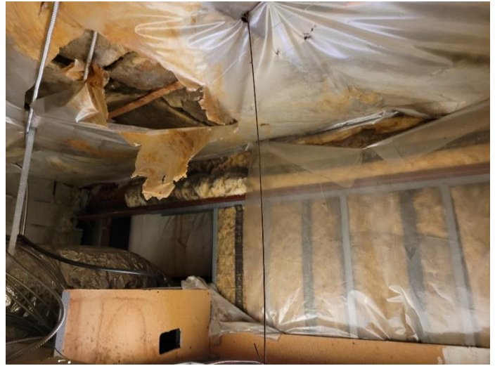
Photo 18 – Mould and Evidence of Moisture
