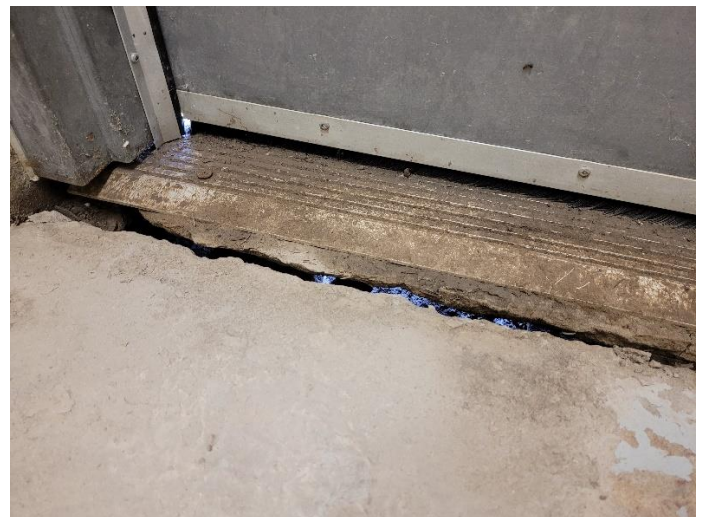
Photo 20 – Damaged Concrete Slab and Open Gap to Building Exterior
