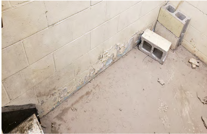
Photo 046 Paint Chipping and Moisture Damage
