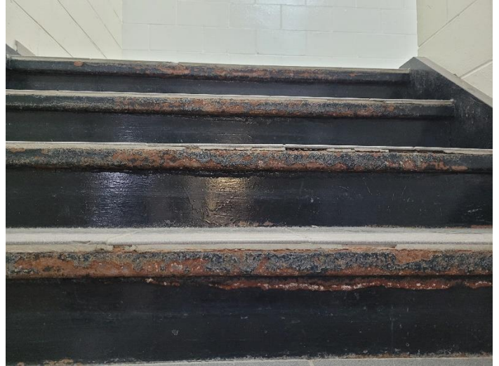
Photo 14 – Corroded/Damaged Stair Treads
