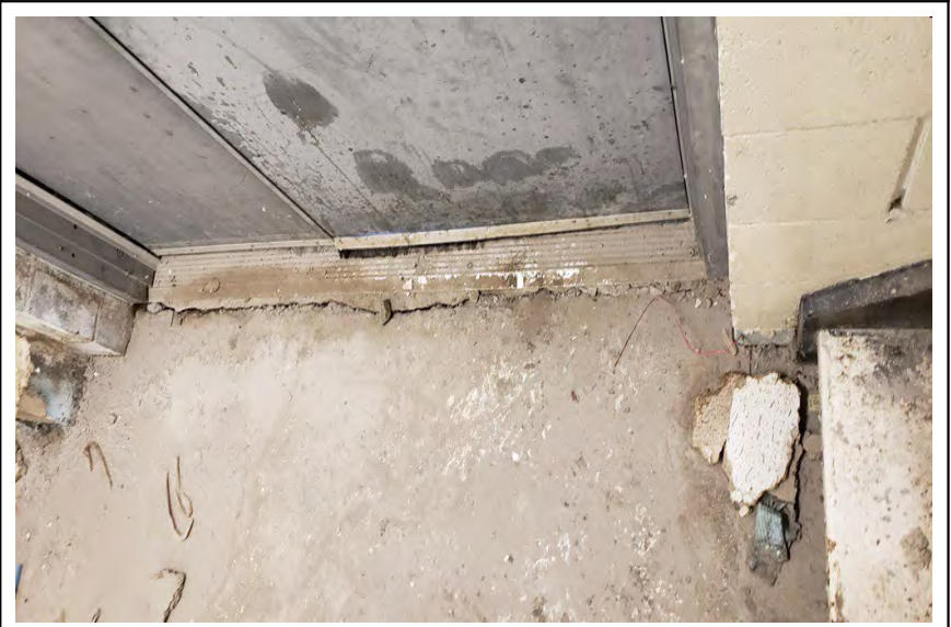
Photo 054 Slab-On-Grade Damage in West-Side Stairwell
