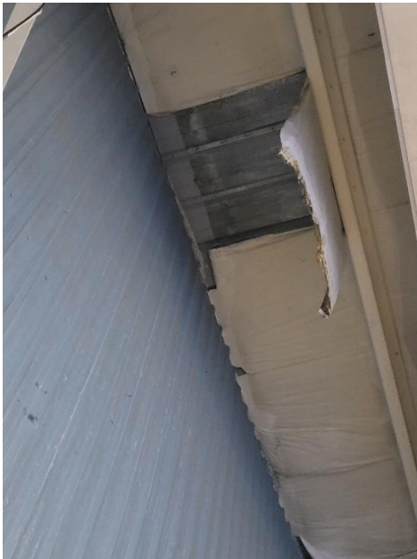
Photo 03 – Damaged Roof Insulation
