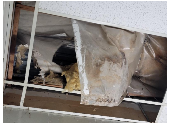
Photo 16 – Damaged Roof Insulation and Evidence of Moisture
