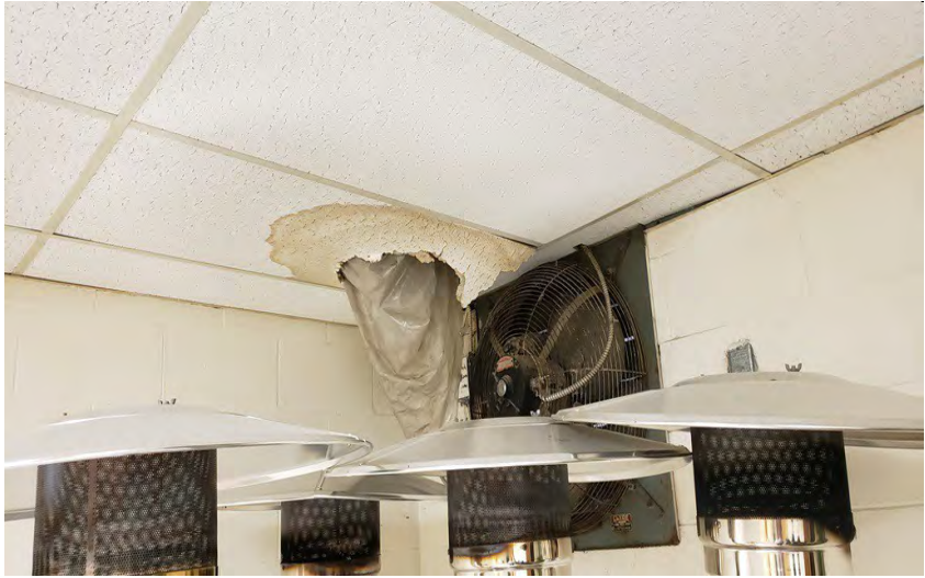
Photo 062 Signs of Moisture Damage
