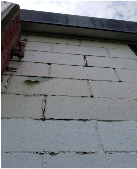
Photo 080 Step Cracking and Paint Peeling
