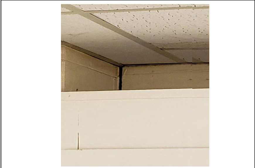
Photo 049 Wall Separation in Second-Floor Storage Room
