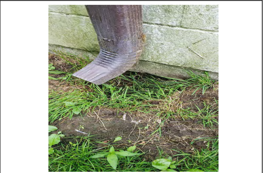
Photo 092 Localized Foundation Wall Damage
