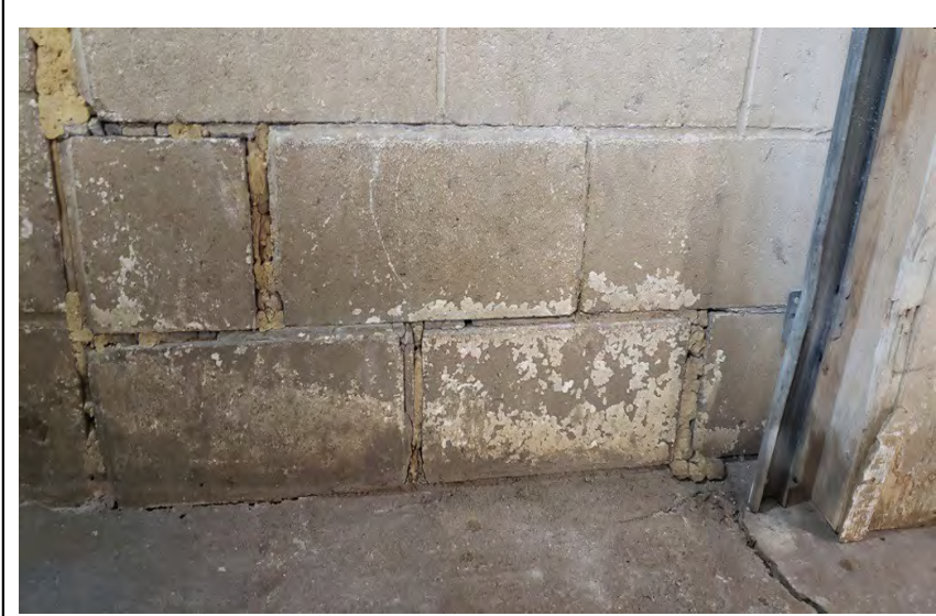
Photo 037 Existing Block Separation Repairs
