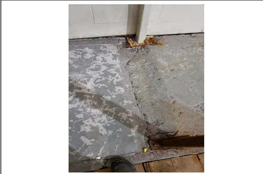
Photo 025 Crack Underneath Mechanical Equipment Stand
