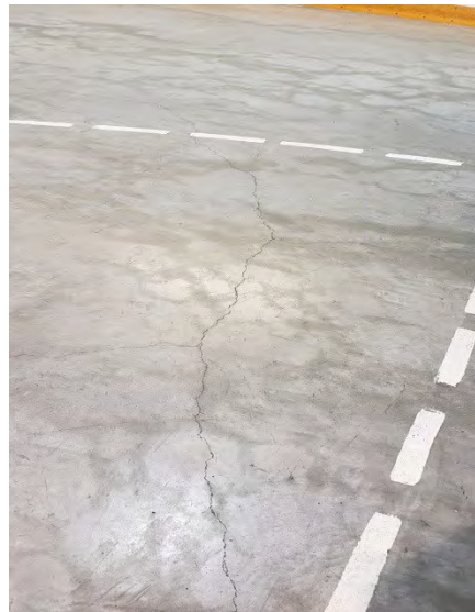
Photo 016 Thermal Cracking on Rink Slab
