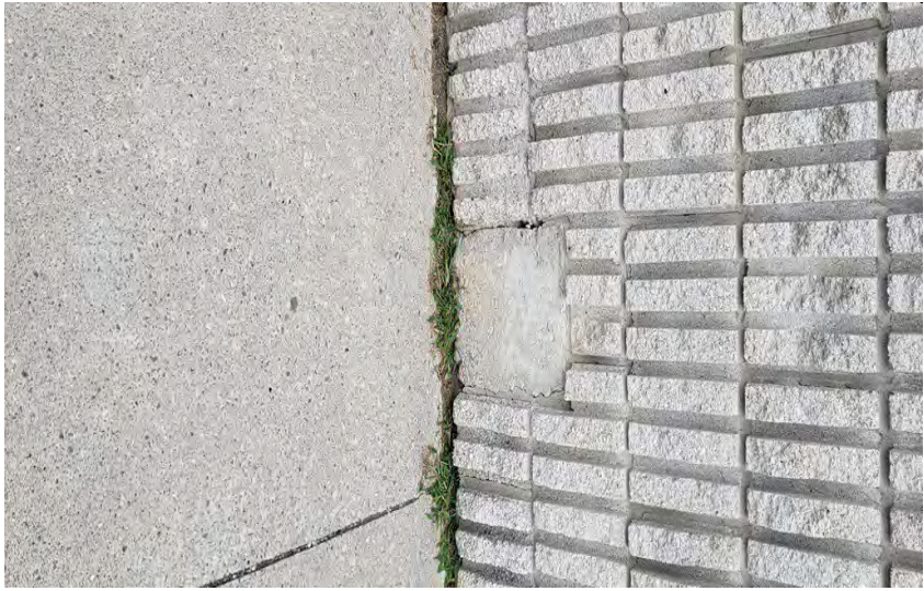
Photo 064 Cracking at Centre Foundation Wall
