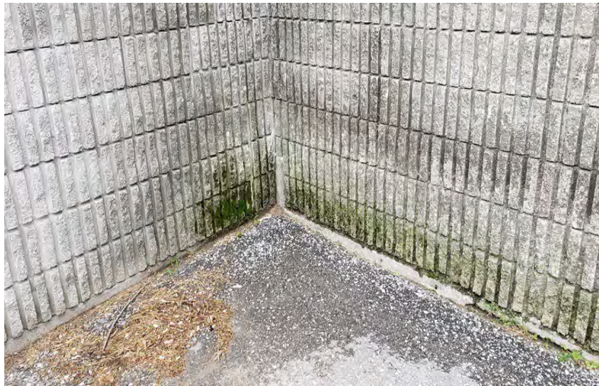
Photo 073 Moss Along East Side Wall
