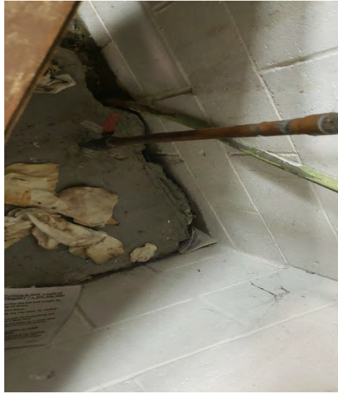
Photo 051 Slab-On-Grade to Wall Separation in Compressor Room
