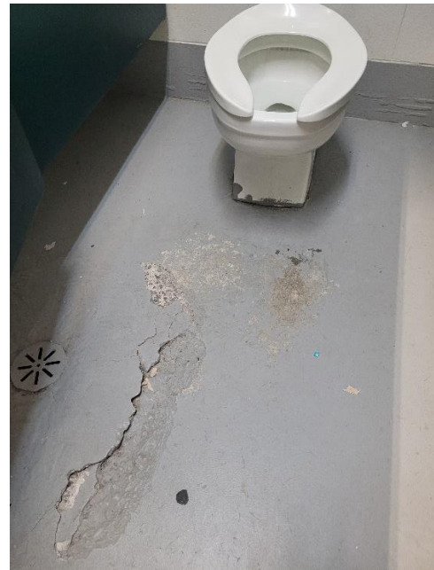
Photo 12 – Damaged Slab in Washroom
