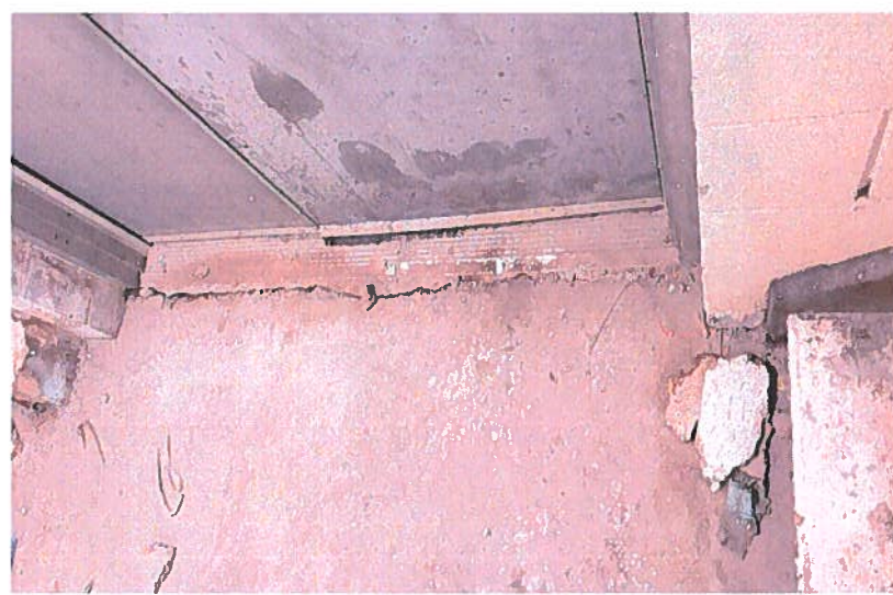
Photo 054 Slab-On-Grade Damage in West-Side Stairwell
