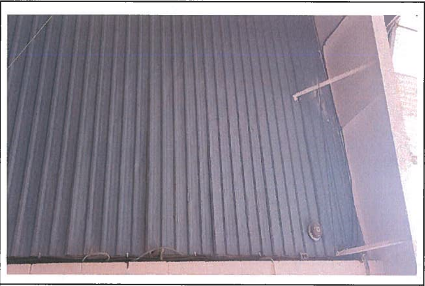
Photo 012 Localized damage to MetalCladding
