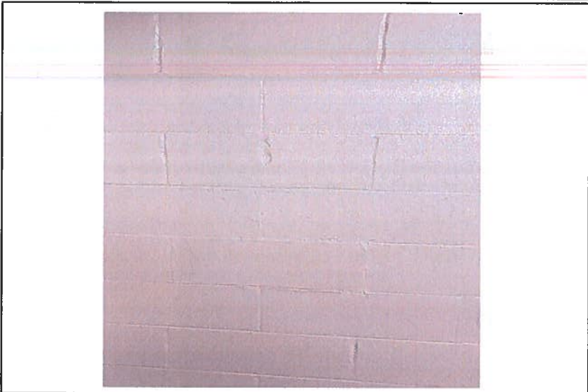
Photo 043 Localized Damage in Changeroom 3
