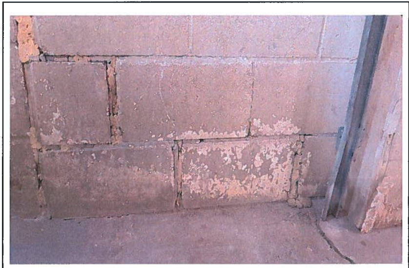
Photo 037 Existing Block Separation Repairs
