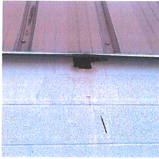
Photo 093 Hole in Masonry Block
