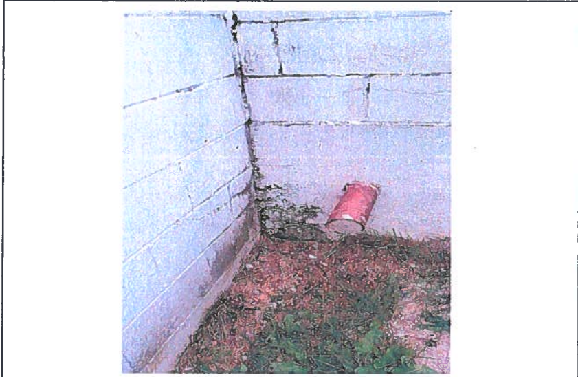
Photo 082 Honeycombing and Mould Growth
