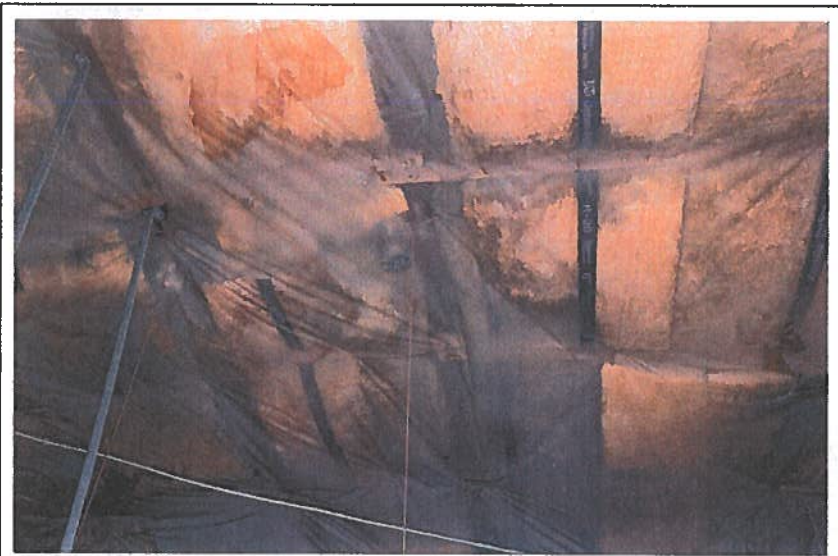
Photo 060 Moisture in Roofing System
