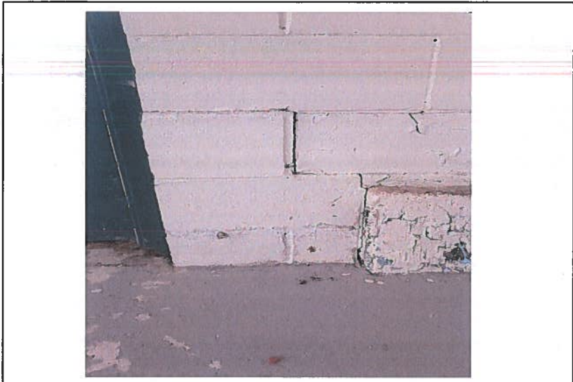
Photo 039 Step Cracking and Damage to West-Side Exit
