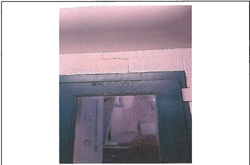
Photo 030 Step Cracking in Lobby
