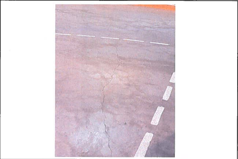
Photo 016 Thermal Cracking on Rink Slab
