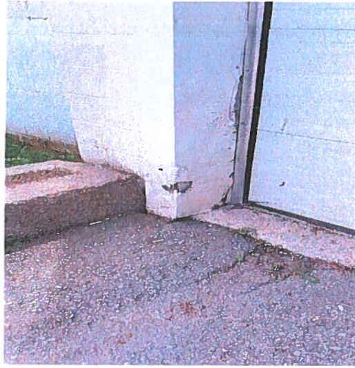
Photo 085 Damage to Garage Door Entrance
