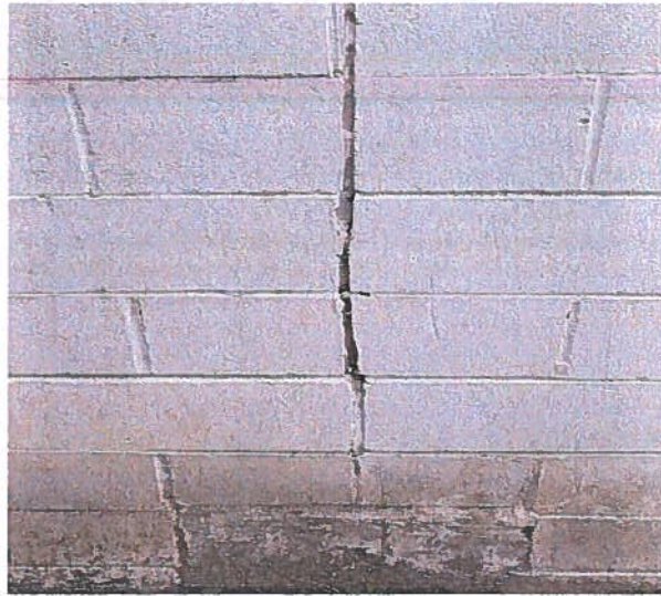
Photo 091 Damaged Wall Joint
