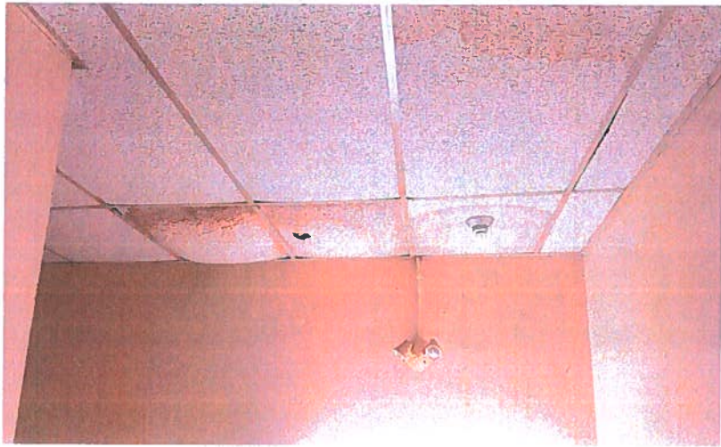
Photo 061 Signs of Moisture Damage
