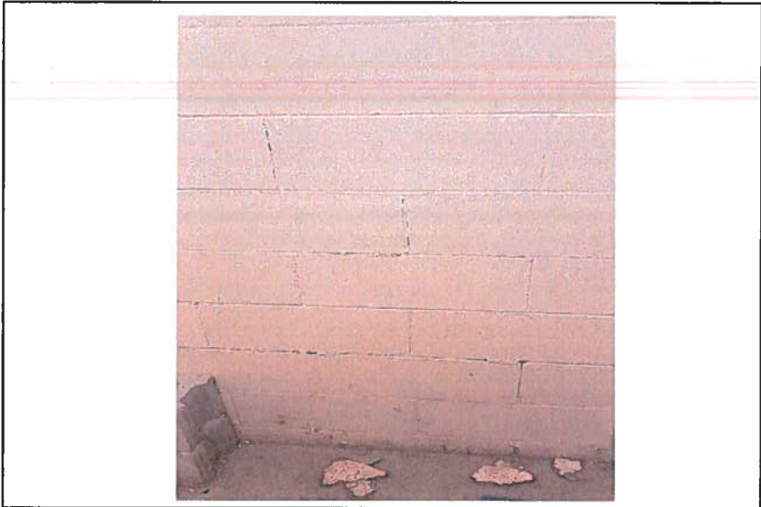
Photo 031 Minor Step Cracking in West-Side Stairwell
