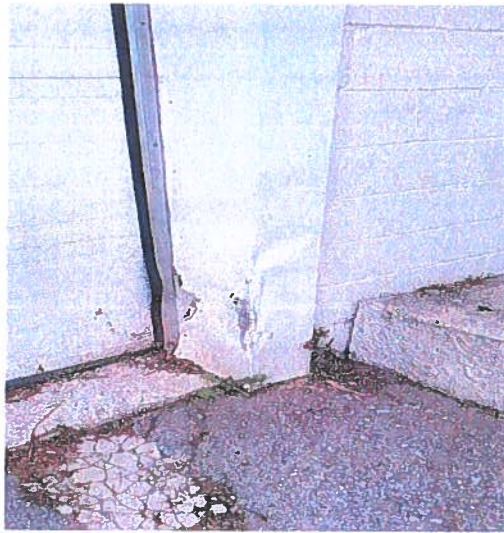
Photo 086 Damage to Garage Door Entrance
