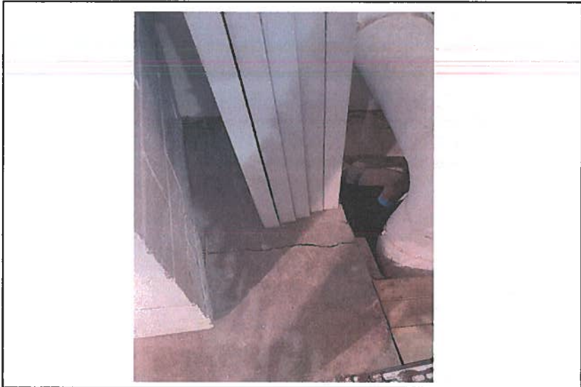
Photo 019 Major Crack in Apron Slab
