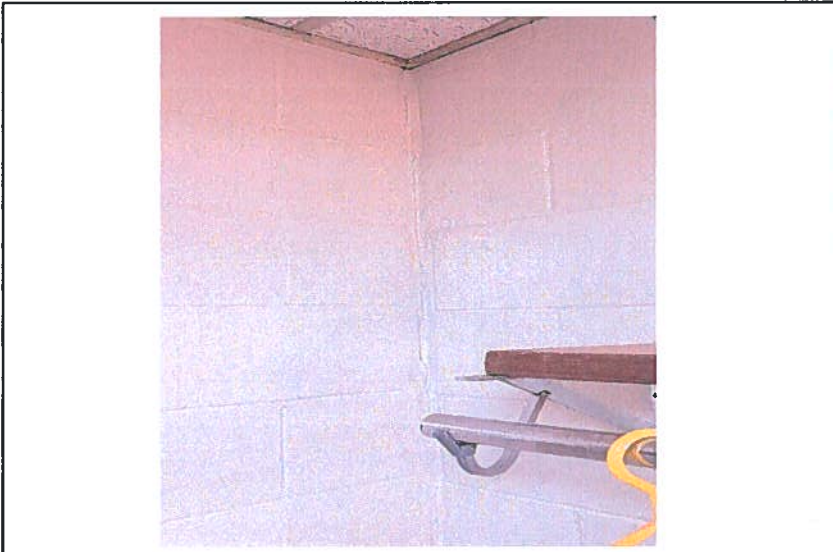
Photo 034 South-Side Stairwell Mortar Joint Cracking
