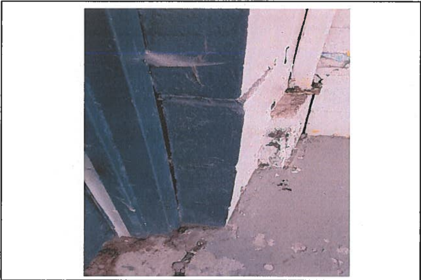
Photo 040 Wall Separation at West-Side Exit
