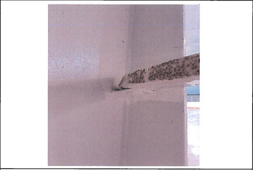
Photo 004 Rust on Frame Brace
