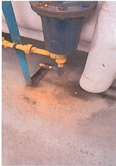
Photo 052 Concrete Staining in Compressor Room
