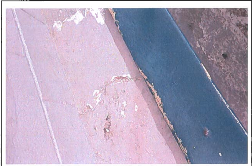
Photo 010 Paint Chipping and Crack on Bleachers
