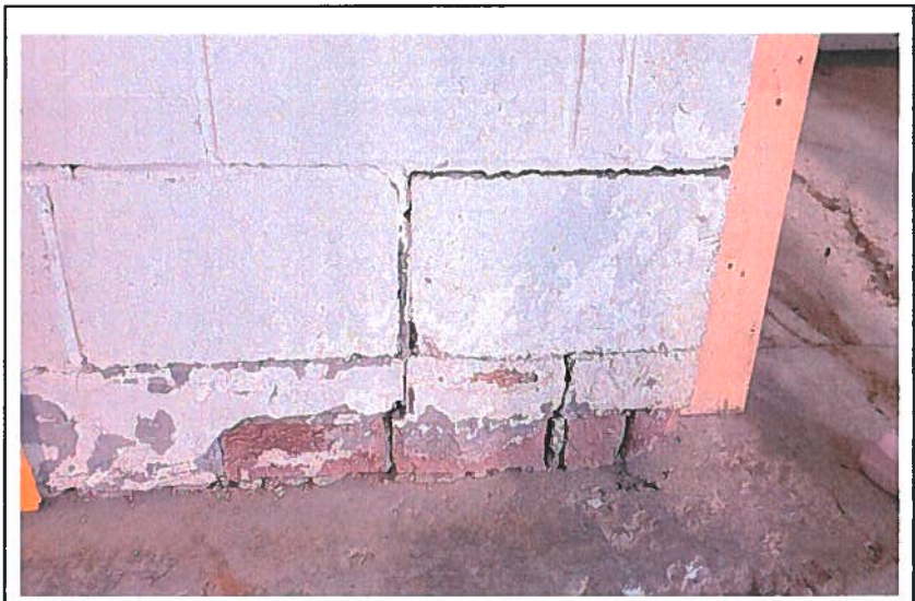
Photo 038 Block and Joint Damage
