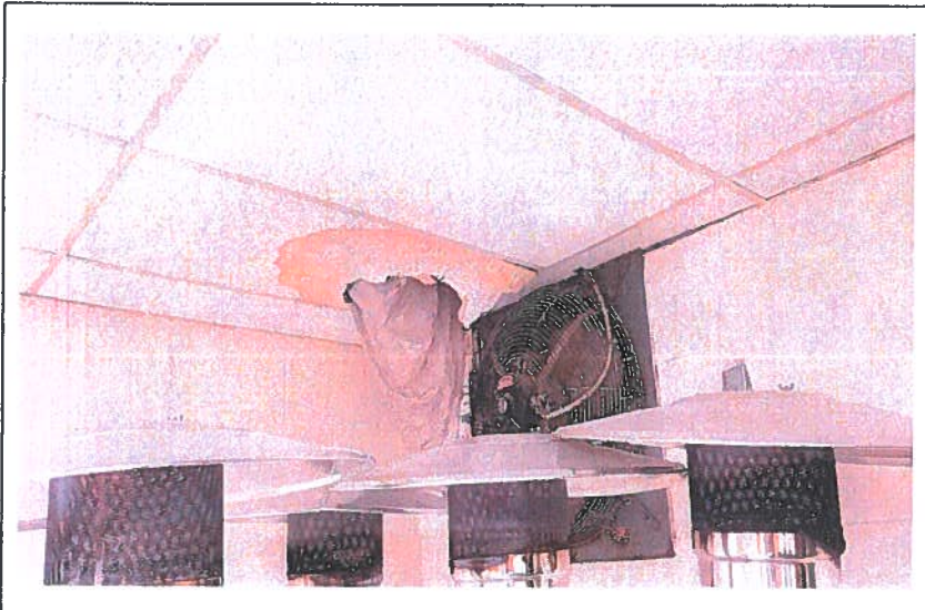
Photo 062 Signs of Moisture Damage
