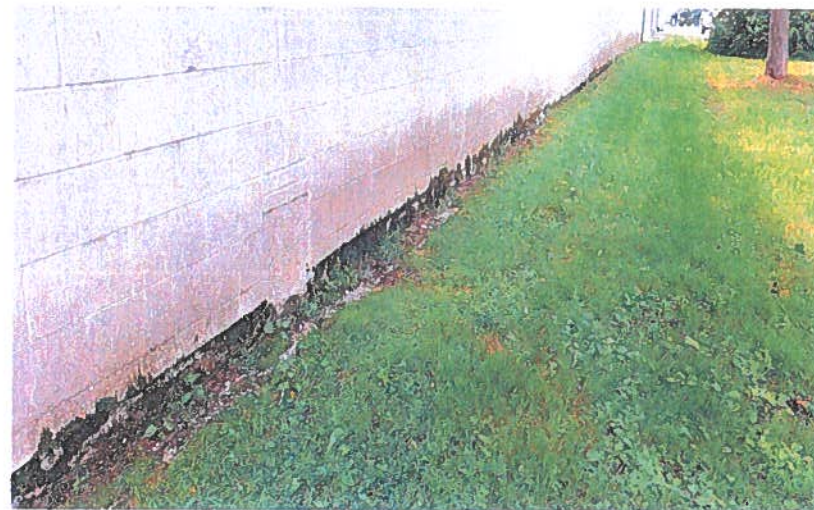
Photo 090 Mould Along West Side
