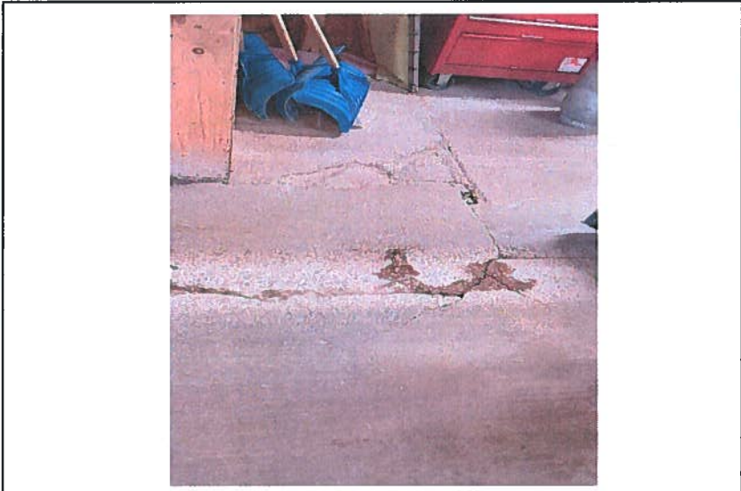
Photo 021 Cracking Starting in Resurfacing Room
