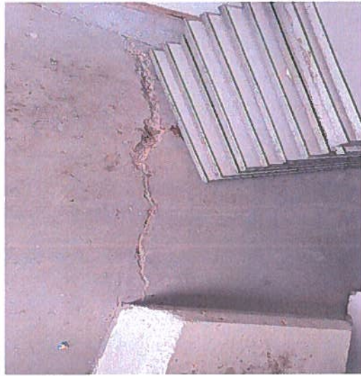
Photo 017 Cracking Outside of Compressor Room
