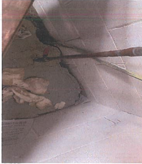
Photo 051 Slab-On-Grade to Wall Separation in Compressor Room
