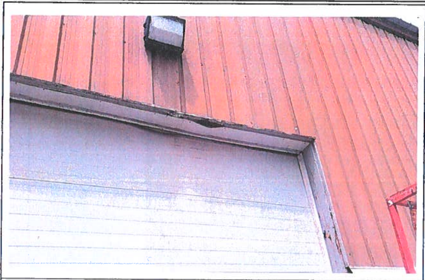
Photo 077 Damage to Garage Door Opening
