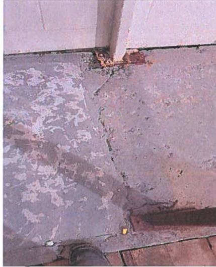
Photo 025 Crack Underneath Mechanical Equipment Stand
