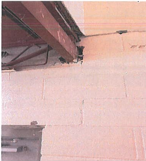
Photo 047 Localized Block Failure
