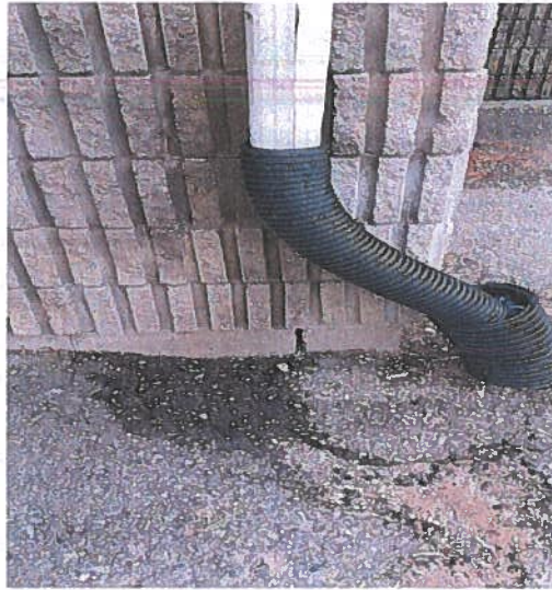
Photo 071 Gap in Foundation Wall
