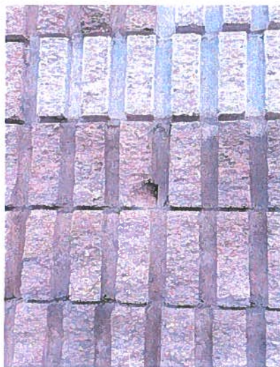
Photo 066 Localized Brick Damage
