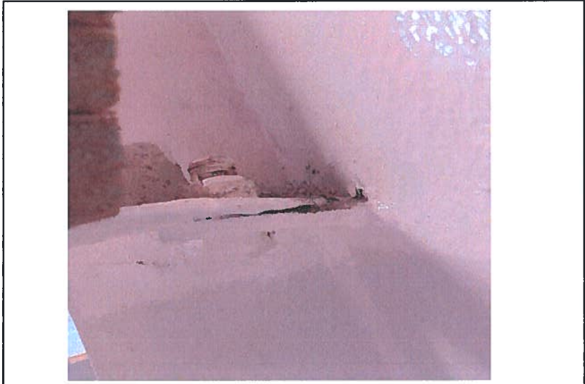
Photo 006 Rusted Bracing Connection
