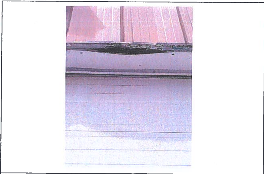
Photo 078 Close Up of Damage Garage Door
