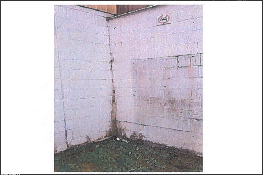
Photo 088 Mould and Moisture on Block Wal
