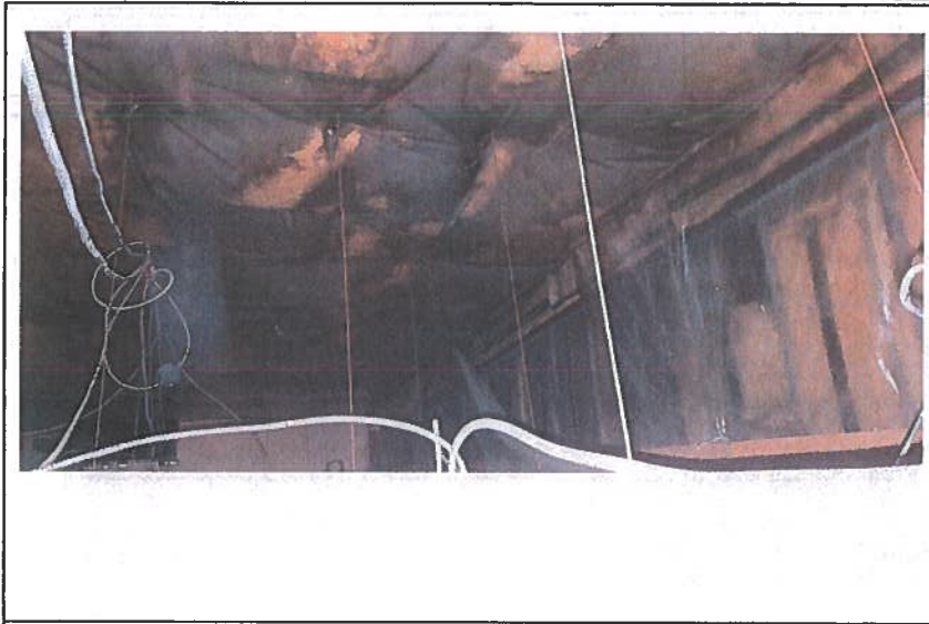
Photo 059 Moisture in Roofing System
