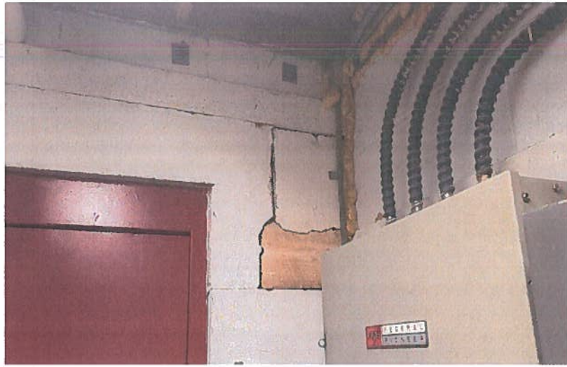
Photo 035 Wooden Block Replacement and Cracking
