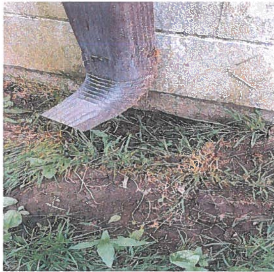
Photo 092 Localized Foundation Wall Damage
