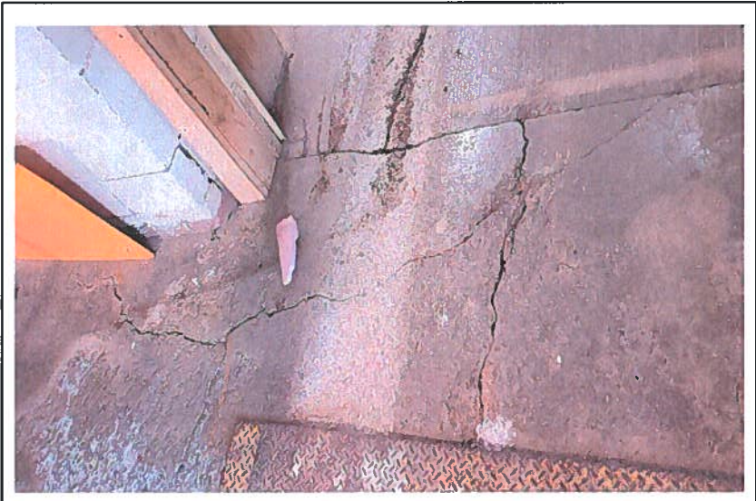
Photo 022 Extents of Resurfacing Room Cracking
