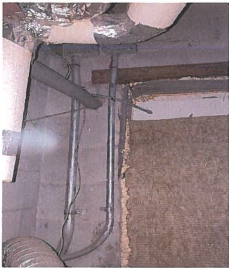
Photo 048 Localized Block Failure
